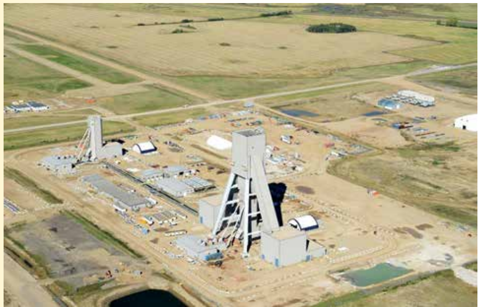
BHP's Jansen Potash Project, located approximately 140 kilometres east of Saskatoon, will enable productivity through innovation and technology.
