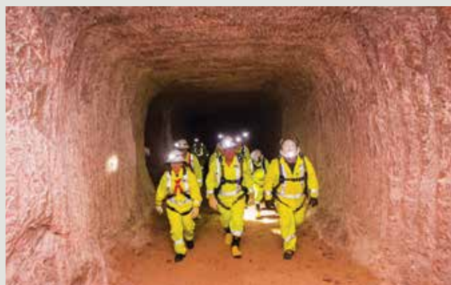
Mosaic's new Esterhazy K3 mine is on target for completion in 2024. The entire complex is expected to be the largest underground potash mine in the world. PHOTO COURTESY OF THE MOSAIC COMPANY.
