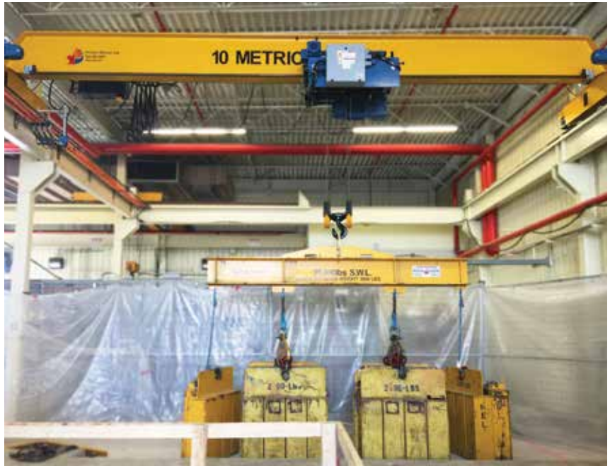
In July of 2017 Kristian Electric was commissioned to load test three new overhead bridge cranes at the Mosaic K2 plant which would be used for maintenance purposes at the new overland conveyor transfer house, part of the K3 expansion project.
