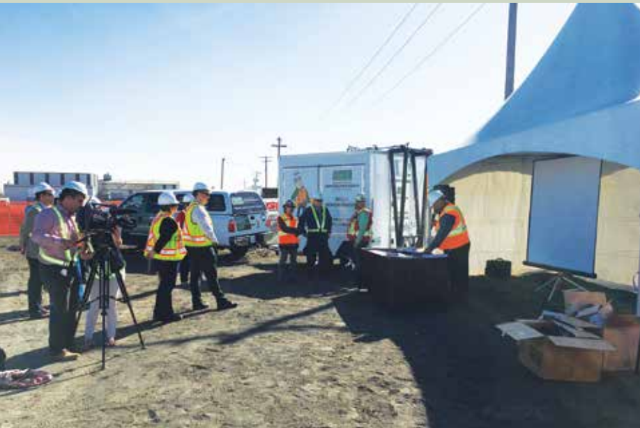
Preparing for official launch at the Graham Construction worksite for the RM of Sherwood Potable Water Treatment Plant.
