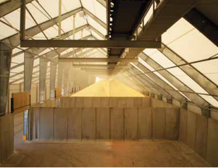
IEI storage bays.
